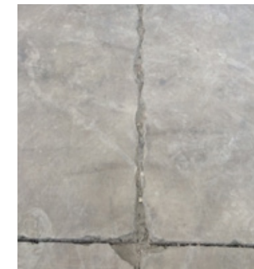
Damaged concrete slab before repair
