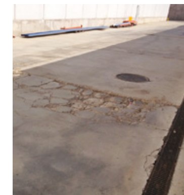
Damaged concrete slab before repair
