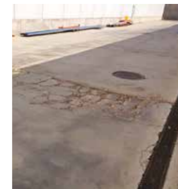
Damaged concrete slab before repair
