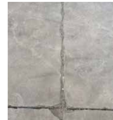
Damaged concrete slab before repair
